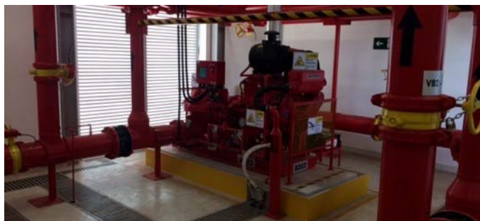
Figura 15 – Bomba diesel (SANDOZ, 2017)
